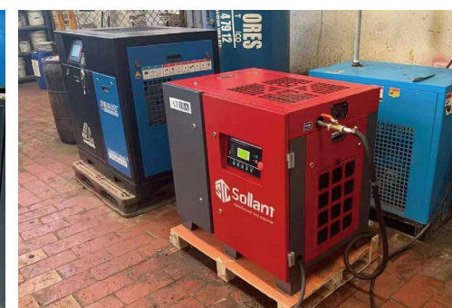
VSD Screw Air Compressor for Rubber Industry in Thailand
