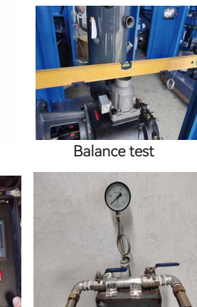
Exhaust pressure test
