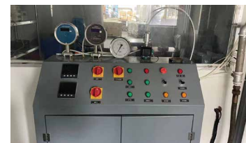
Air dryer pressure dew point detection
