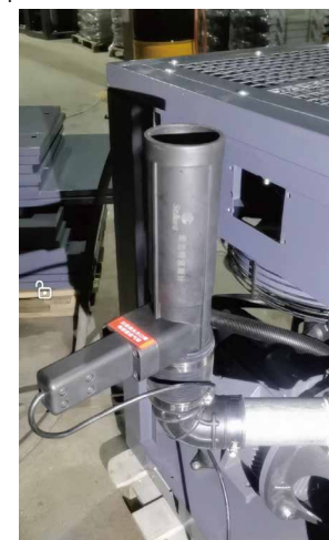
Measure air compressor inlet flow
