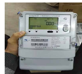
Measure air compressor total power
